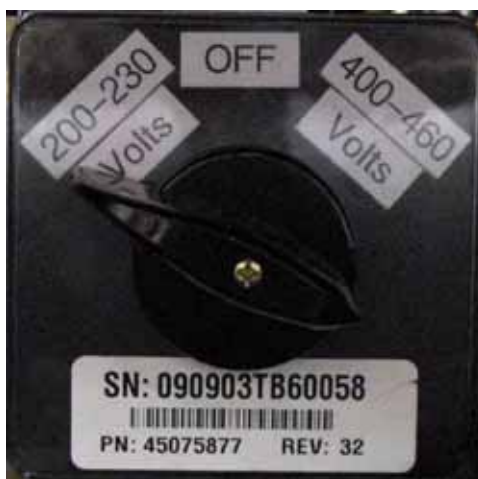
Figure 1-3: Main AC input voltage switch
