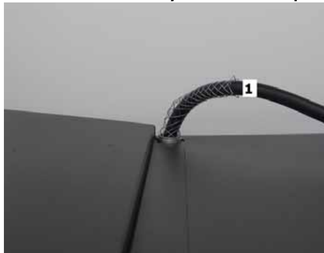
Figure 1-7: AC Power Cord from facility circuit breaker panel, top right rear
